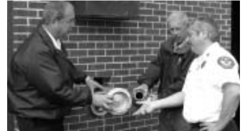
Retired Chief Bob Buhs, Orland Fire Protection District, Acting Chief Dan Wysocki and Jack Nance, Local 281 Training Instructor, check out the standpipe outside the Arthur Granat Sr. Training Facility in Orland Park.
