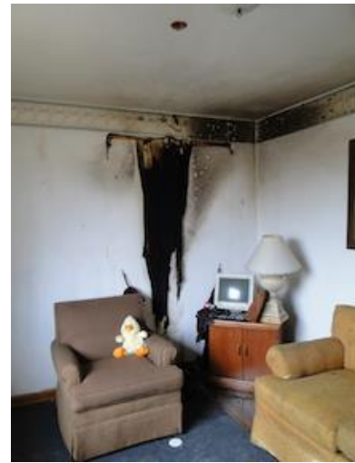
Post-Burn: Fire Sprinkler- Protected Room
